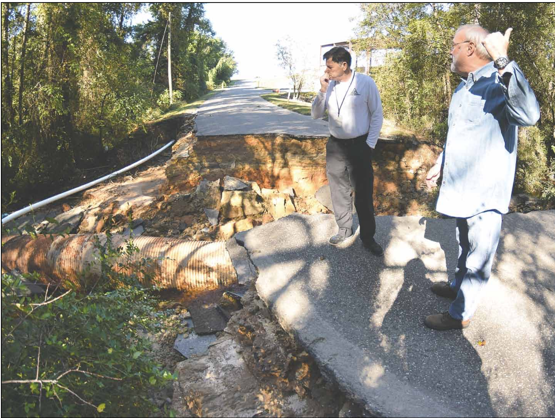
Hoke Sheriff's Emergency Management Director Freddy Johnson (left) and Hoke Solid Waste Director Don Russell plot a workaround to get garbage collection going again. The county's transfer station is on the other side of this break in the road. And so are two sorely needed garbage trucks. (Ken MacDonald photo)
