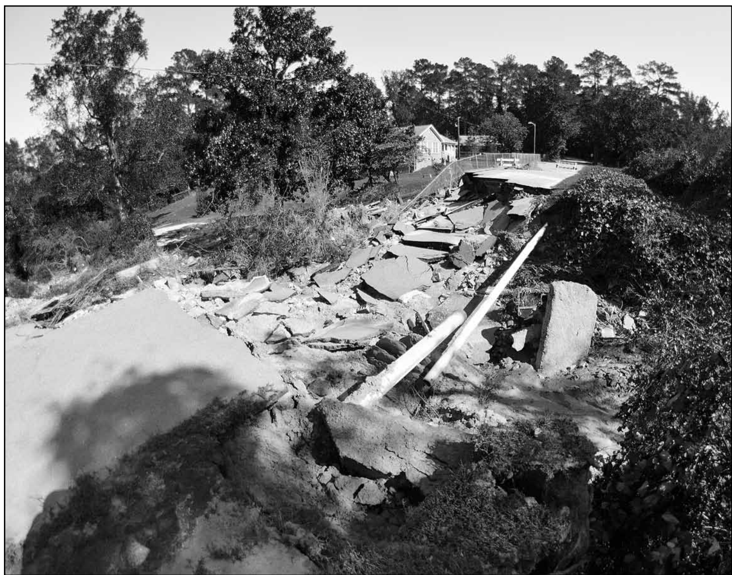
Oakwood Avenue, behind old Johnson Concrete, was destroyed at its lowest point. (Ken MacDonald photo)
