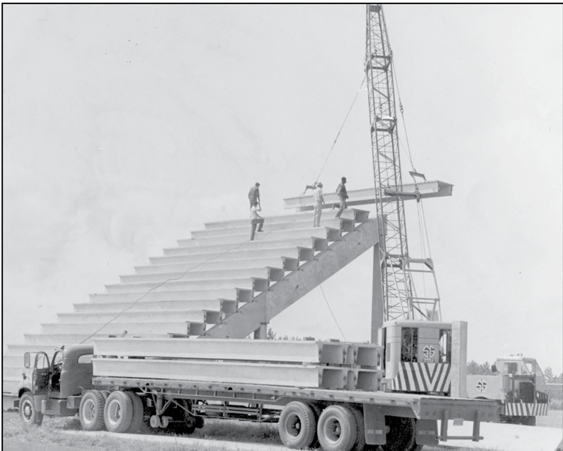
With the hoisting of this last row of bleachers, the stadium reaches its one-sixth mark. The structure is expected to be complete in 10 days.
