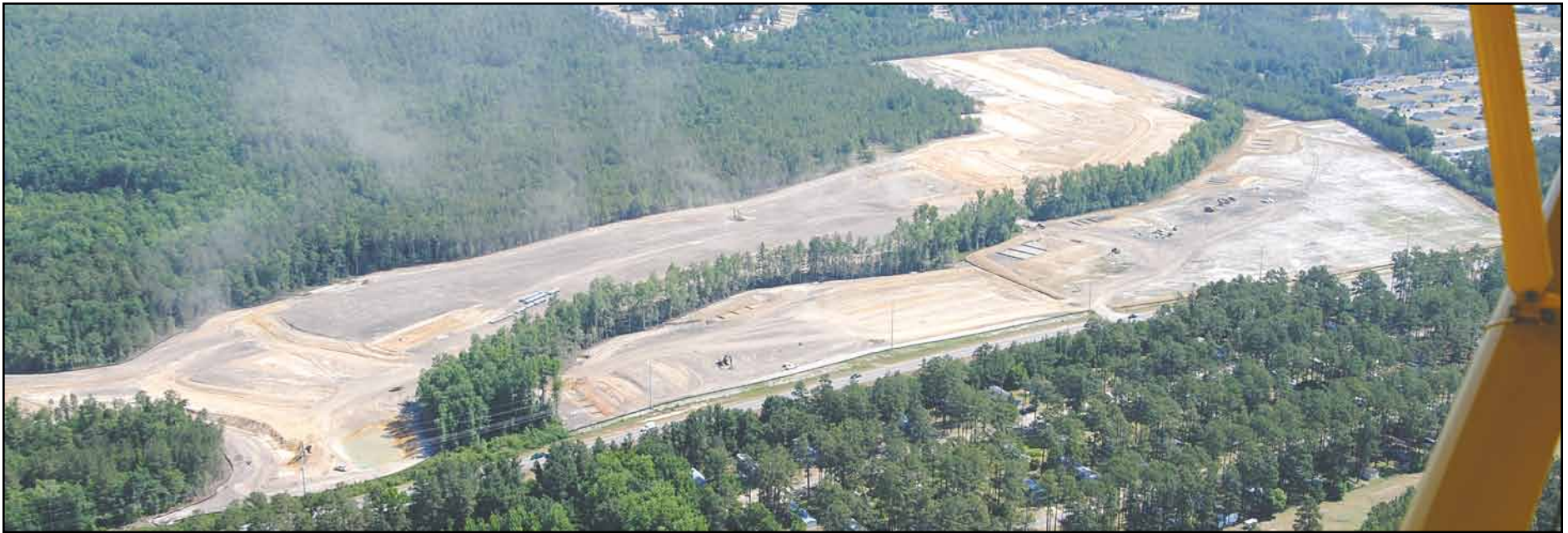
Construction is underway on a housing complex along U.S. 401. With 4 lanes, and now other infrastructure improvements, the highway continues to attract growth.
