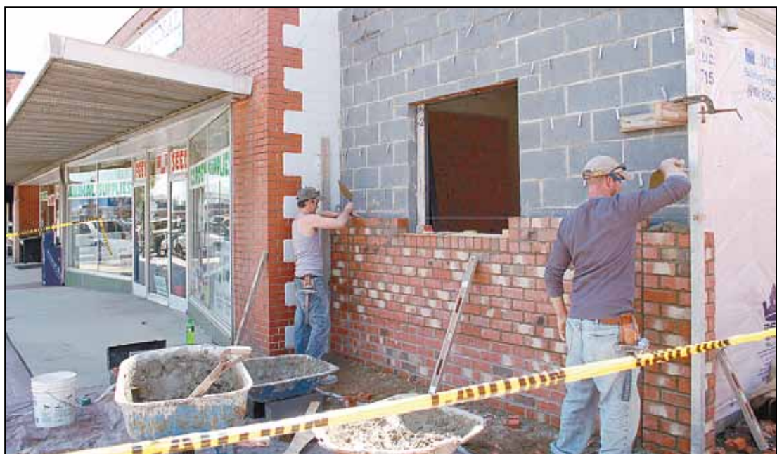
Workers with Henry's Masonry build what will be the take-out window for the Home Food grill and café.
