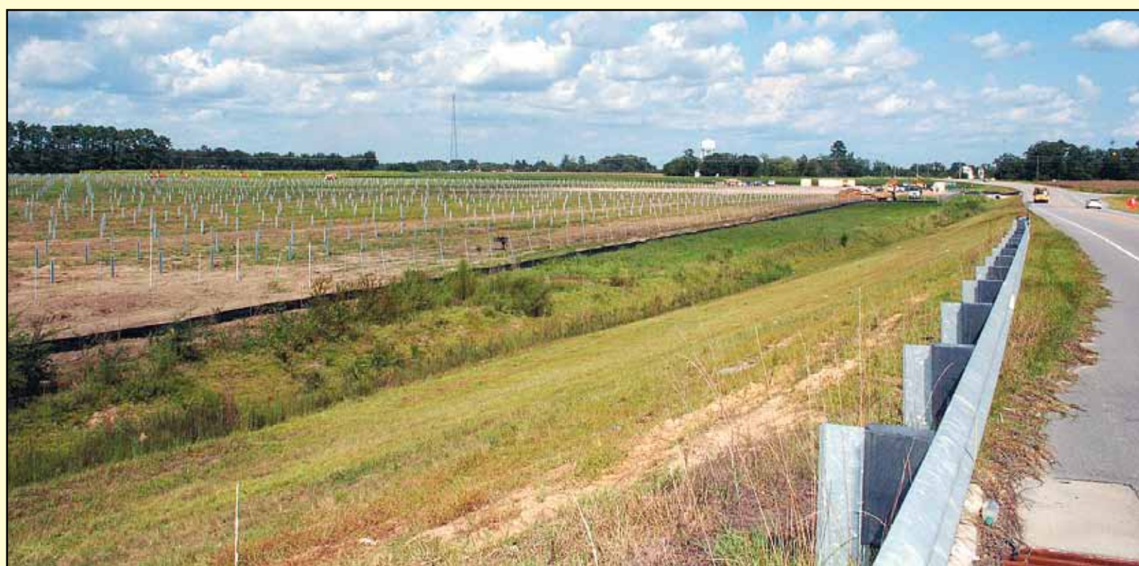
Support poles go up at a solar farm located at St. Pauls Rd. and East Palmer Street. The poles will soon hold solar panels. (Catharin Shepard photo)
